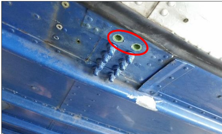
Figure 2. Outboard Bolts Removed and Location of Inspection, RH Wing Root
