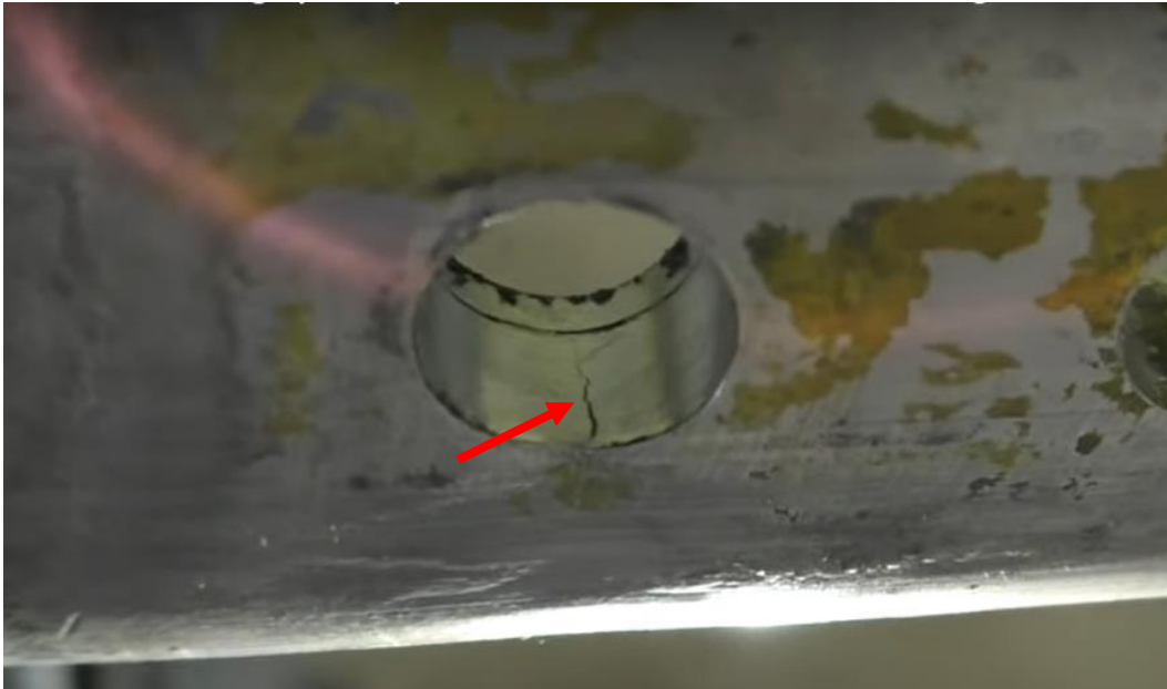
Figure 6. Example of Cracks Intersecting Bolt Hole PA-32-300, 5,319 hours TIS
